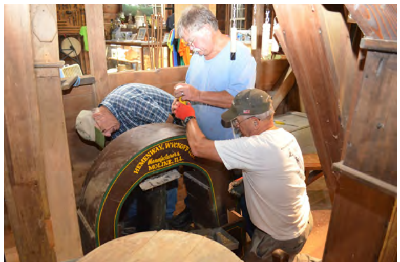
Larry Driscoll, Brian Bentley and Hank Mann are preparing to remove the smutter's top air duct so they can reach the beater chamber below. No, you don't want to see what we found inside.
