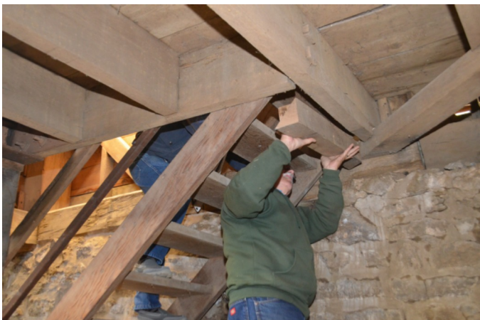
Above Dick and Clarence are test fitting the new support beam for the basement steps.
